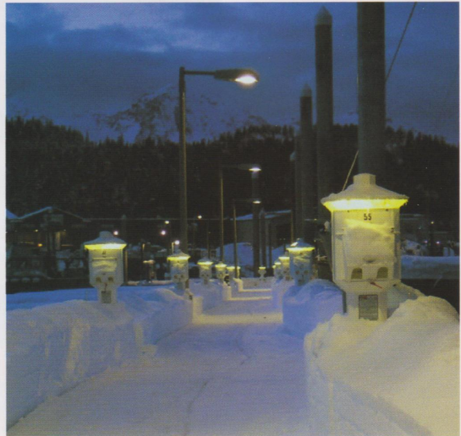
Above: Lighthouse Power Pedestals, Cordova Marina, Alaska
